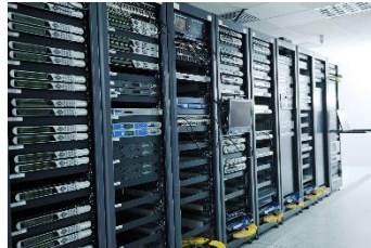
Data center B
