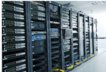
Data center B
